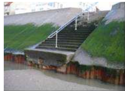
March 2006: new threat to the dyke
